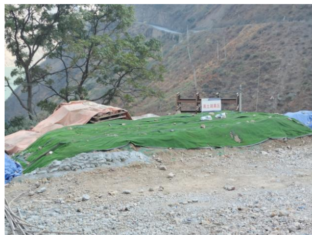
18 标段斯古溪隧道进口表土堆放场堆放不规范
